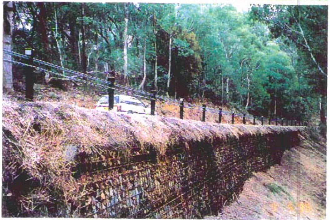
Briten Wire Rope Safety Fence installed at "Reflector" corner on the Alpine Way - one of the many reconstructed sections of the road.
